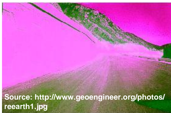
Source: http://www.geoengineer.org/photos/reearth1.jpg Fig. 2.6.7 Retaining wall - Reinforced wall constructed as a mitigation measure.
